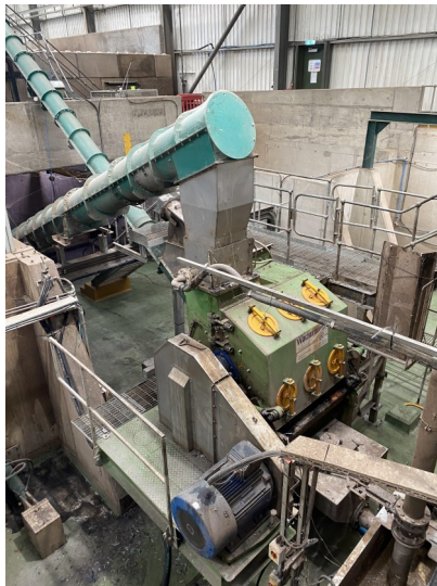
2. The food bags are fed into a macerator (via the big green pipe) which minces them finely. The result is sieved - the plastic waste goes up the little green pipe and .....
