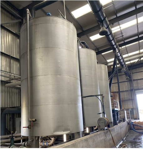
5. (Above) Using excess heat from the gas engines, the digestate is pasteurised at 70 degrees for one hour to eradicate harmful bacteria.
